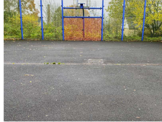
Faded line markings
