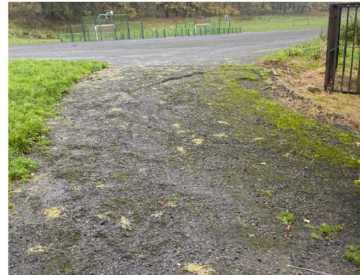
Footpath connection in poor condition
