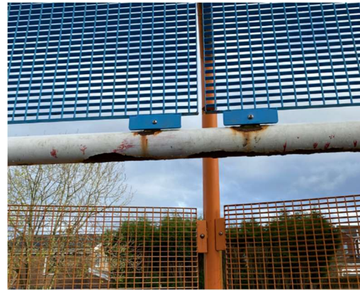
Goal posts have rusted
