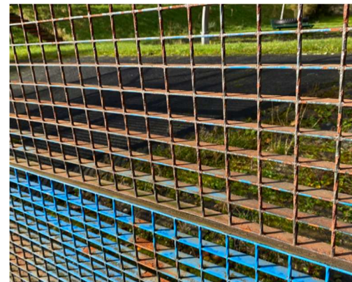
Fence is rusted
