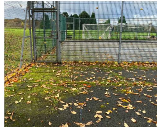
MUGA surface in poor condition
