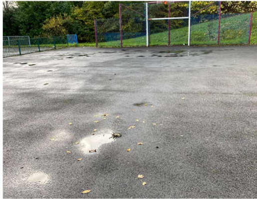
Faded line markings
