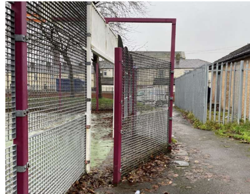
Narrow entrance restricts disabled access
