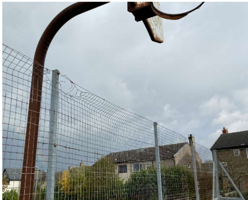
Sections of fence in poor condition
