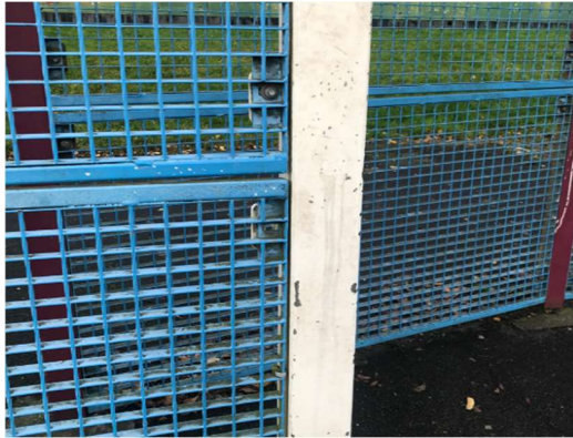
Bolt missing in fence
