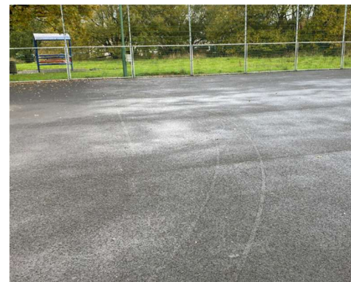
Faded line markings
