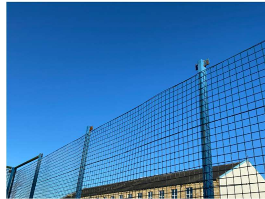
Top rails on fence missing
