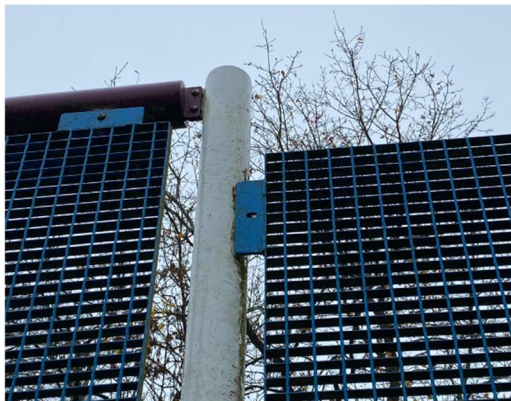
Bolt missing from fence panel
