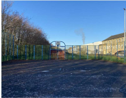
Faded line markings
