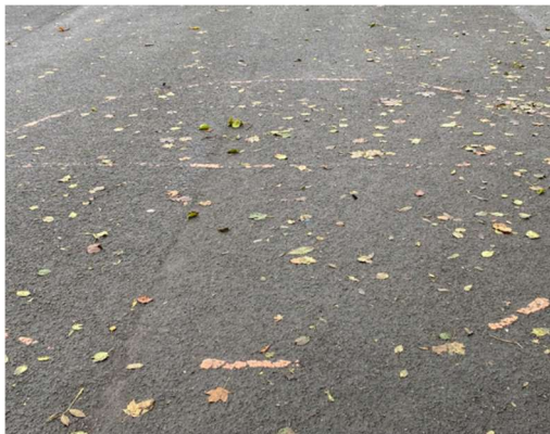
Faded line markings
