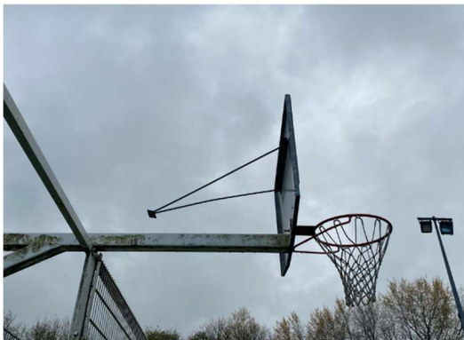
Basketball backboard detached from fence
