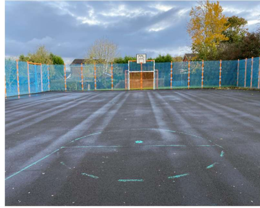
Faded line markings
