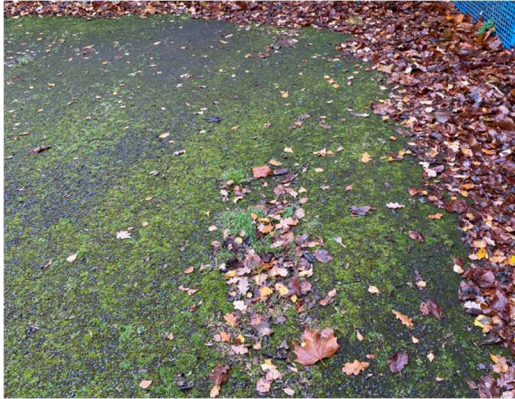
MUGA surface in poor condition
