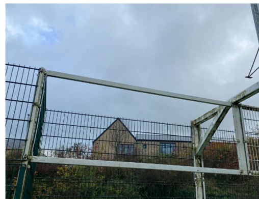
Missing fence panel
