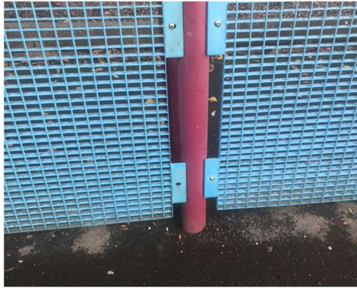
5 No. bolts missing from fence panels
