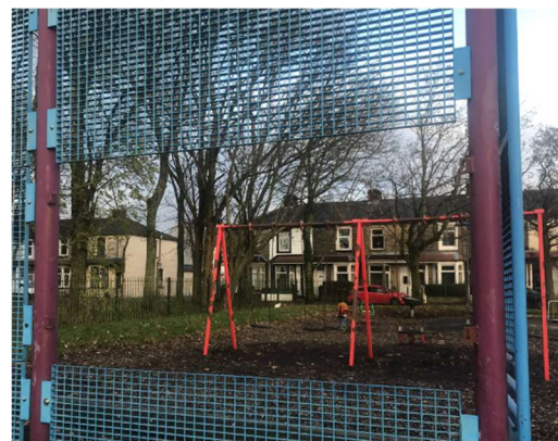
Missing fence panel
