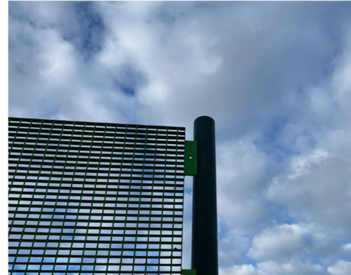
4 No. bolts missing on fence
