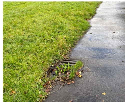
2 No. blocked gullies
