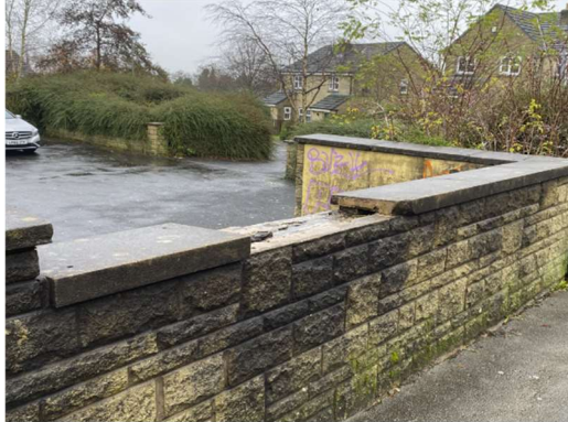
Missing coping stone
