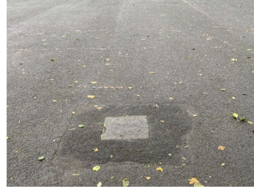
MUGA surface in poor condition
