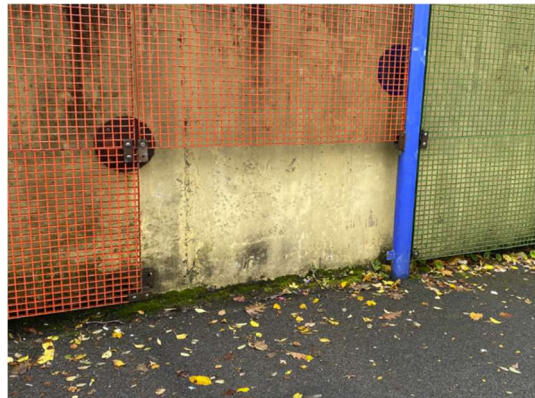
Missing fence panel
