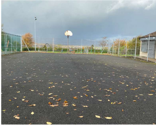
Faded line markings
