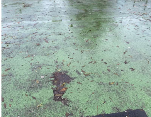
MUGA surface in poor condition
