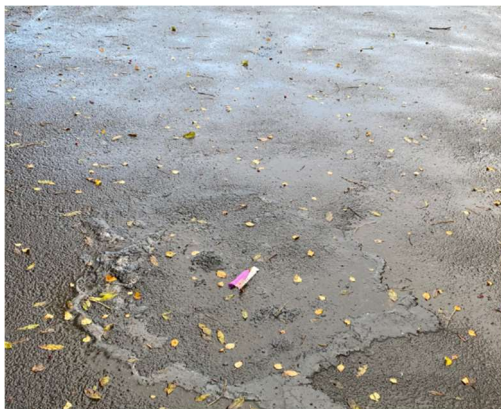
Damaged MUGA surface
