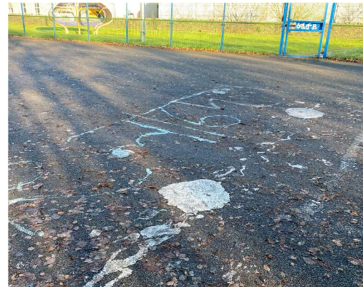
Paint on MUGA surface
