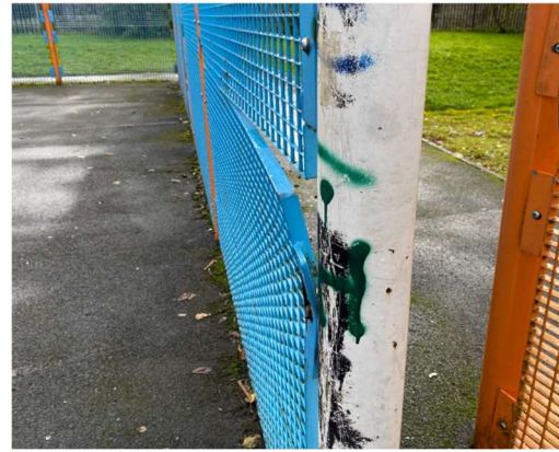
Fence panel bent outwards
