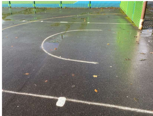
Line markings starting to fade
