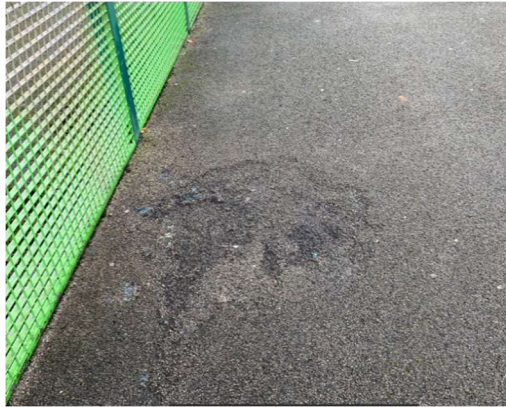
Damaged MUGA surface
