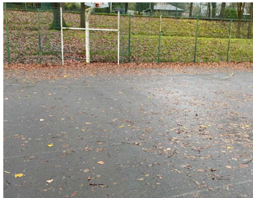
Faded line markings
