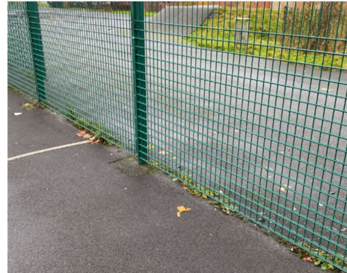
Weeds along fenceline
