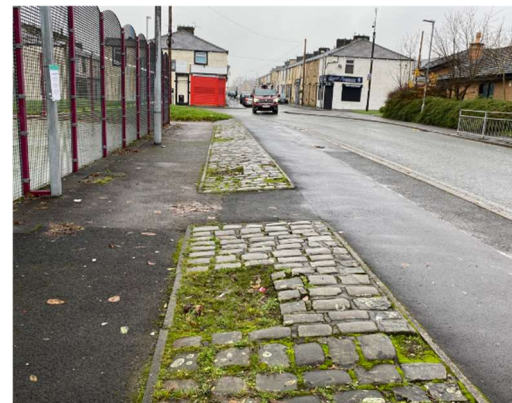
Voids at former tree pits/missing setts
