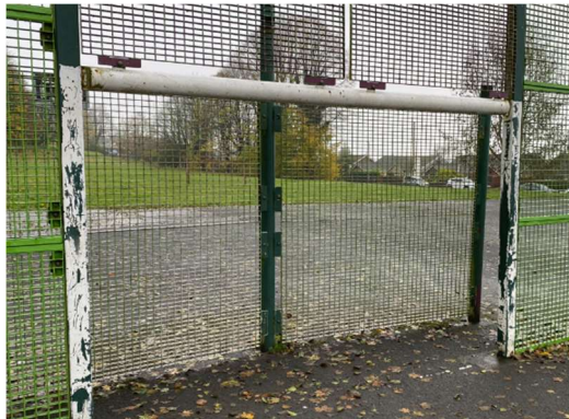
Rusted/scuffed goal posts
