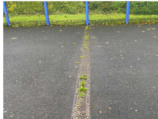
Blocked ACO drain
