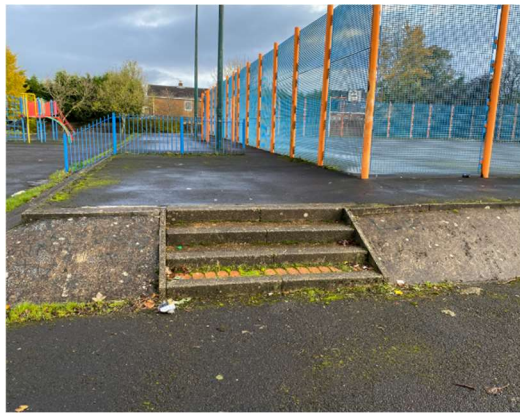
Stepped access restricts disabled users
